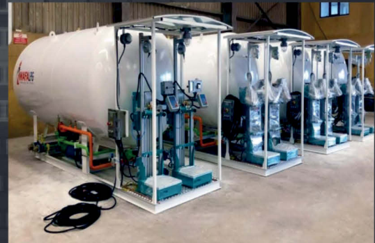
LPG SCALES GAS FILLING CYLINDER SKID AND PLANTS
